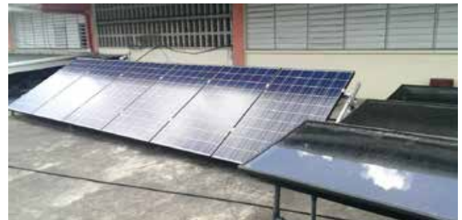
The solar PV panels and solar stills installed on the roof of the Parvati Girls' Hindu College.
